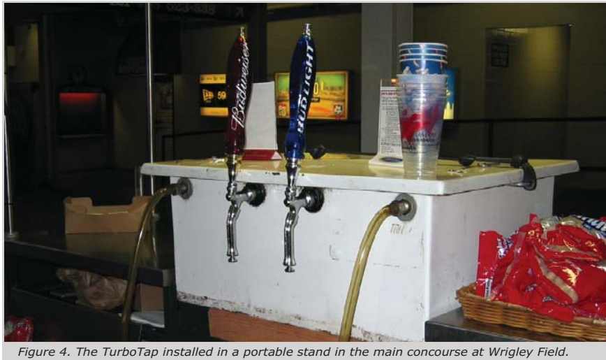
Figure 4. The TurboTap installed in a portable stand in the main concourse at Wrigley Field.
